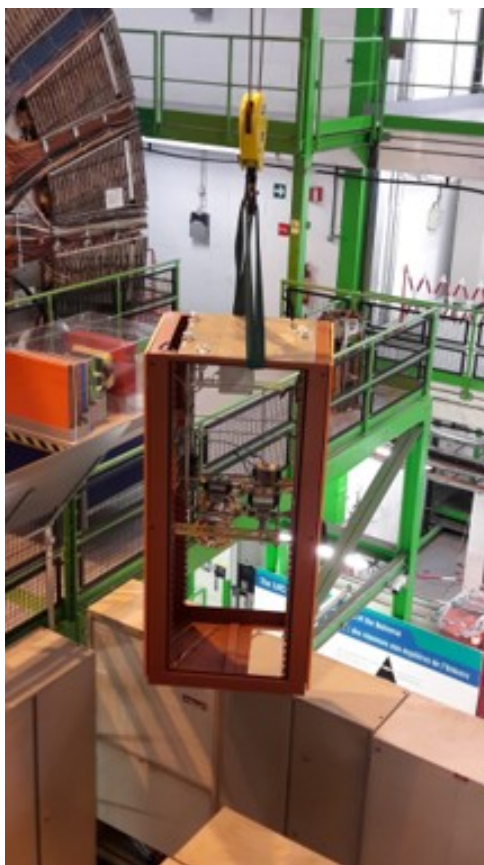
(A) Distribution rack in experimental cavern
