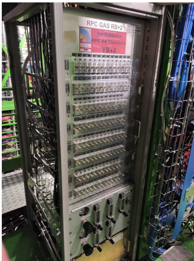
FIGURE 4.9: CMS RPC barrel distribution rack in UXC
