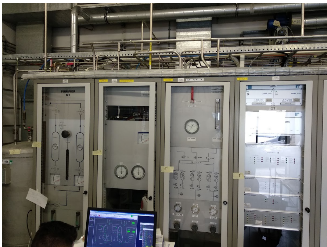
FIGURE 3.2: Racks and high-pressure buffer to be recuperated from LHCb SG.
