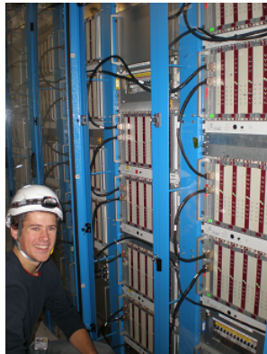
Figure 3.9: Me in front of one of the power-supply racks
