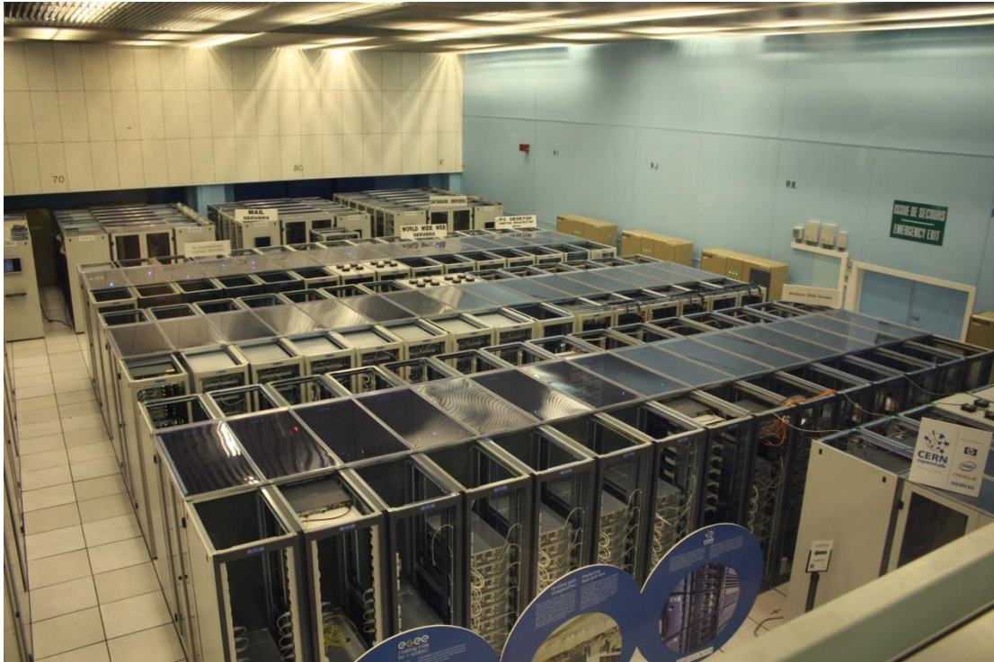
Figure 1-16: CERN data centre
