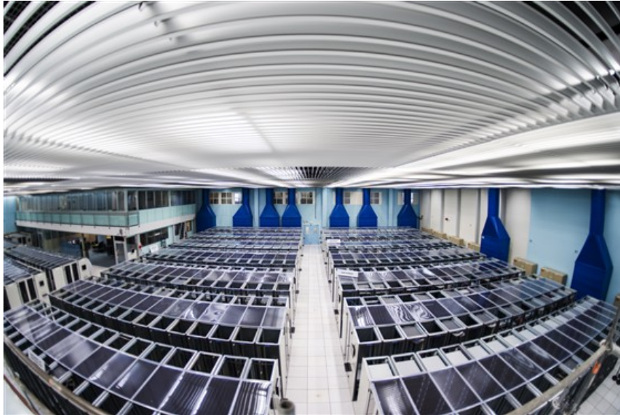
Figure 2: CERN Main Data Center.
