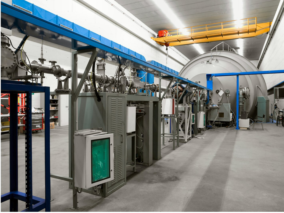
Figure 6.6: The output Tandem accelerator vacuum pipe: the void pumps, as well as the quadrupoles magnetic lenses, which let the beam focused along the beam axis, are visible.
