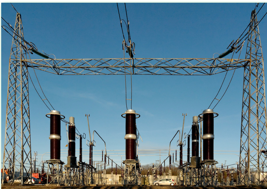
An electrical installation on the CERN site.
