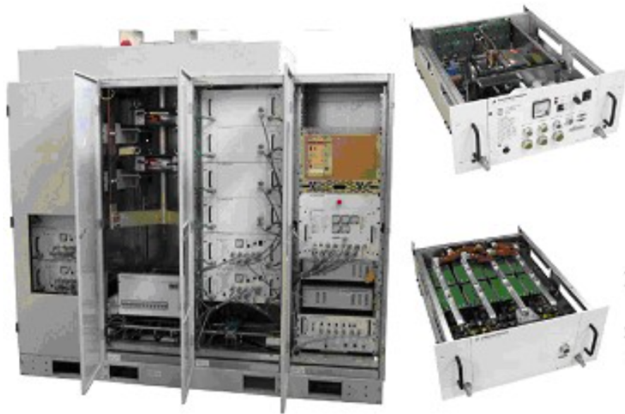
FIGURE 2.9: LHC quadrupole power converter [32].
