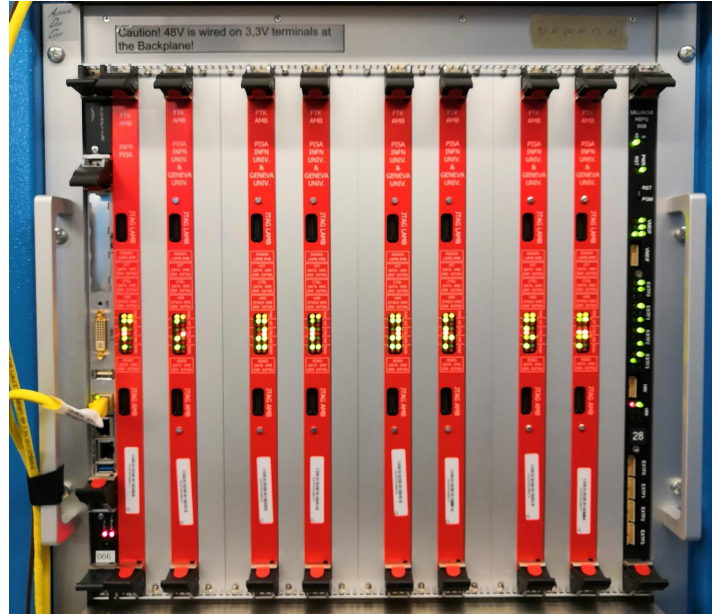
Figure 4.22: Picture of one of the VME crate used for the reduced configuration cooling tests. The crate is load with 8 PUs, one SSB (slot 21, black board), and the Single Board Computer. In order to avoid the dispersion of the air flow from the missing slots, blinds have been used (metallic covers on the slots where the boards are missing).
