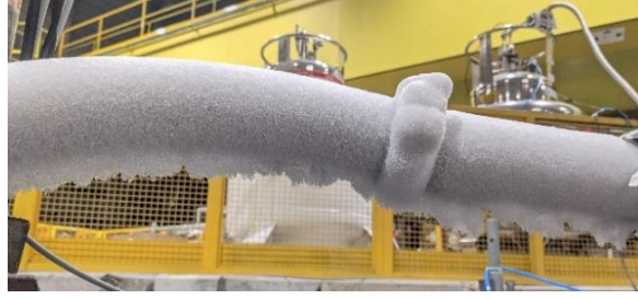
Figure 4.17. Frozen GHe recovery line during a cold test in December 2020. The desublimated ice indicates a cold GHe temperature.
