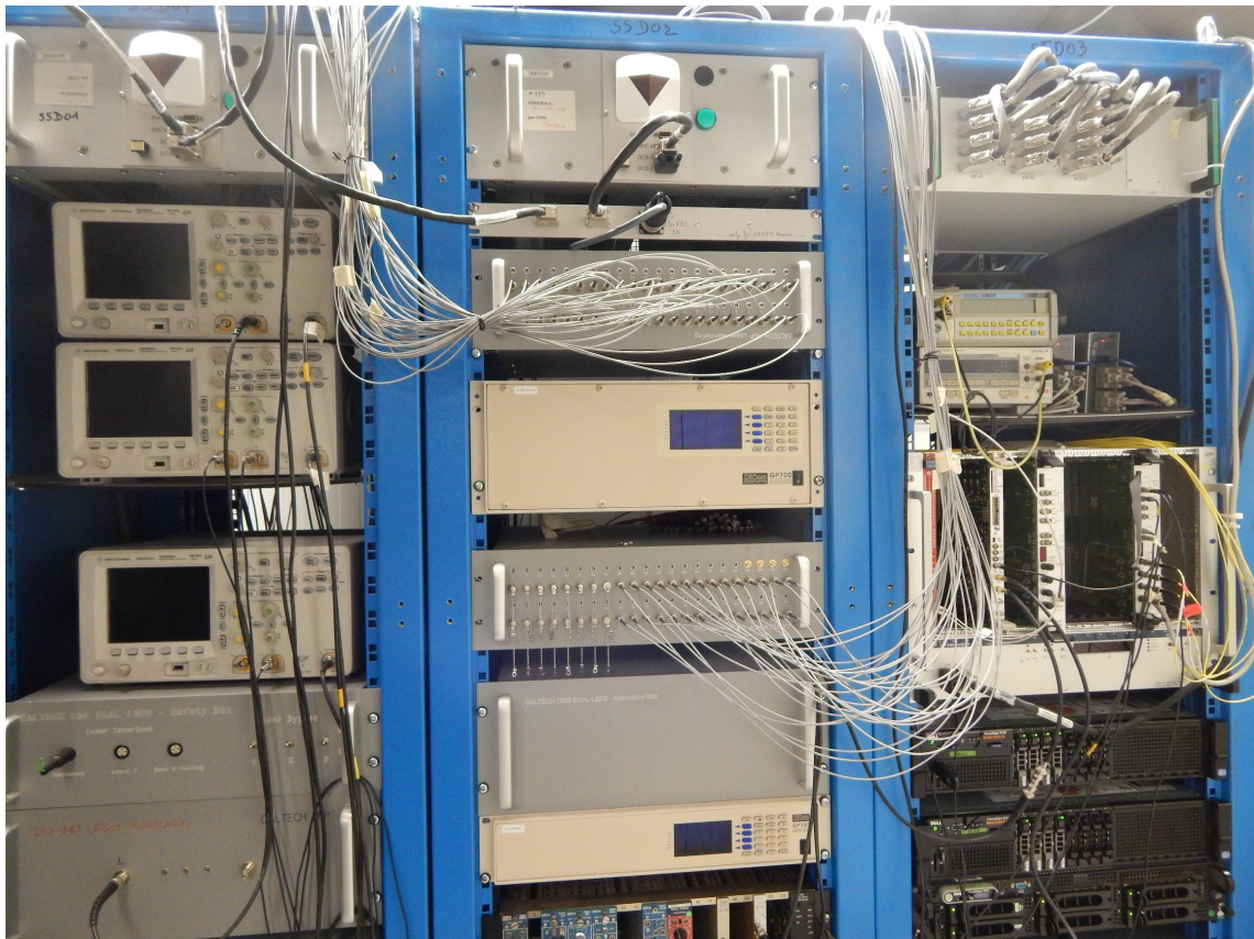
Figure 4.25: The general view of the laser monitoring system in the laser barrack after "SpyBoxes" installation.
