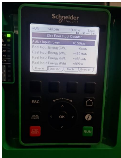
Figure 5 Variable Frequency Drive (VFD)
