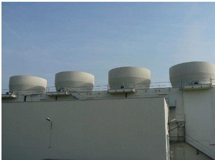
Figure X – Cooling Towers at CERN
