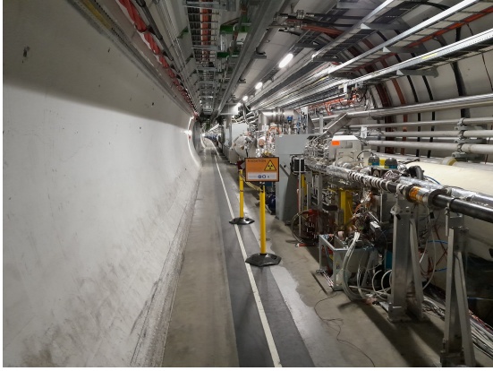
Figure 17: Picture of the far station of the AFP detector on A-Side in the tunnel. The NIM crate lies on the floor of the LHC accelerator tunnel.
