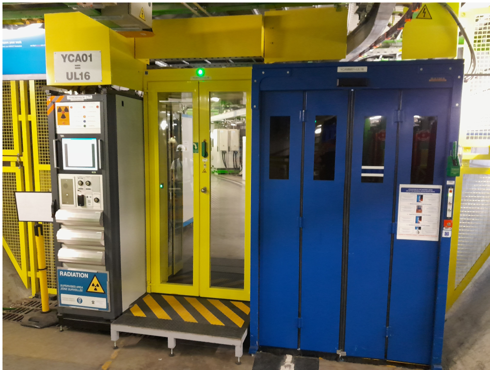
Figure 16: An access door to the LHC tunnel.
