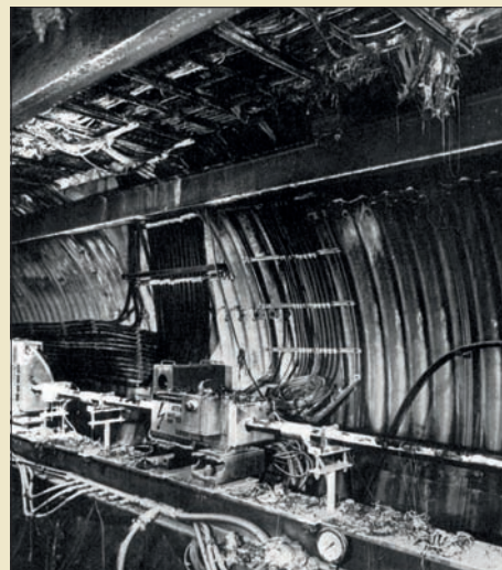
Fire damage in the outer PS tunnel.
