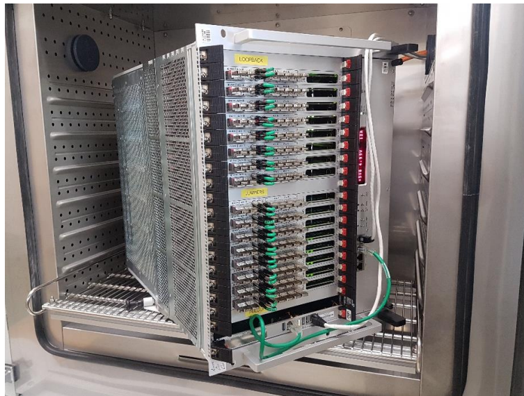
Figure 3.7: Fully equipped VME crate inside the climatic chamber
