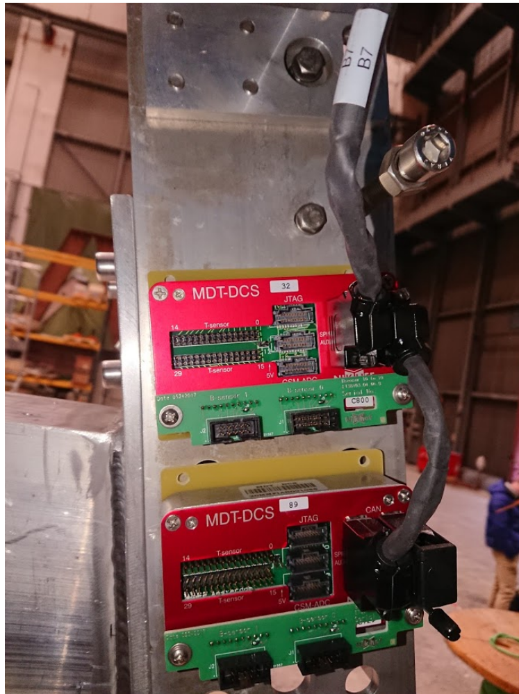
Figure 3.36: MDM modules installed on NSW spokes.
