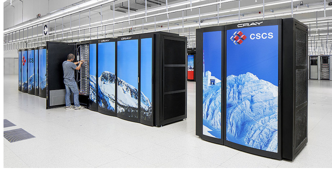
Figure 2.21: A system engineer working on CSCS Piz Daint [151].
