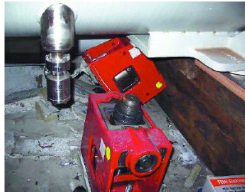
Figure 2: A broken magnet support.
