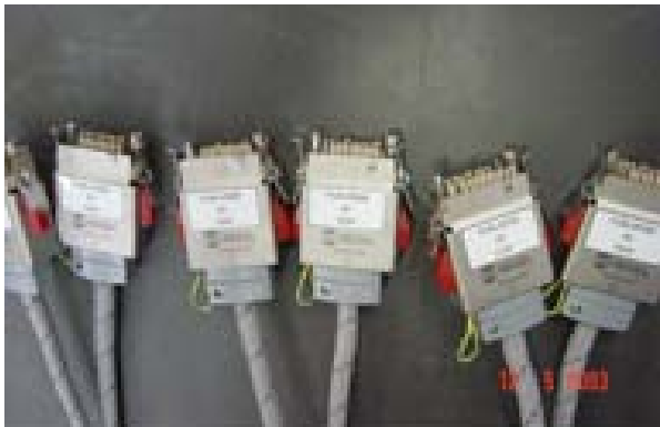
Figure 3.7: High-voltage cable connectors.
