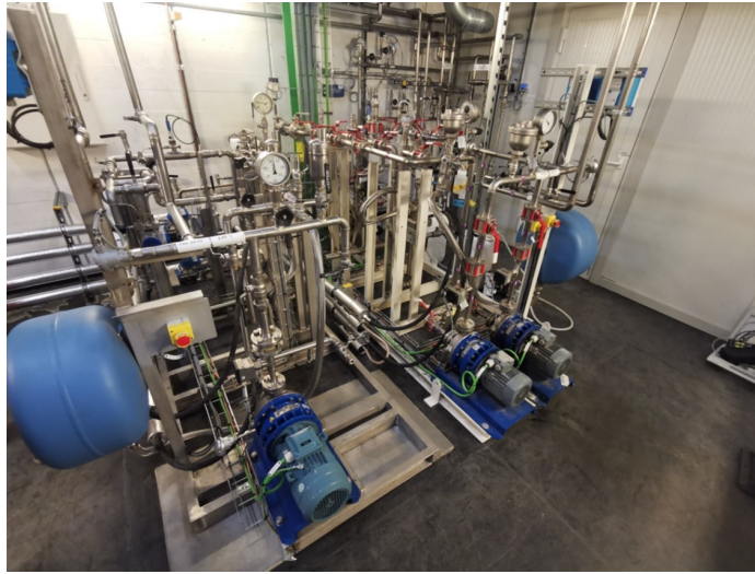
Figure 2.12: Moderator water skids.
