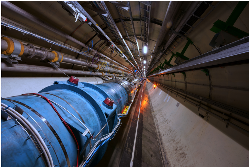
Figure 2: Large Hadron Collider UHV pipes.
