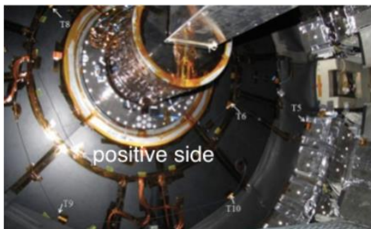
Figure 2: Bulkhead FBG Monitoring System on The Positive Side
