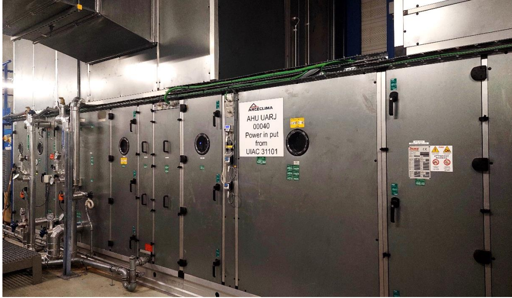
Figure 4: HVAC system in building 311
