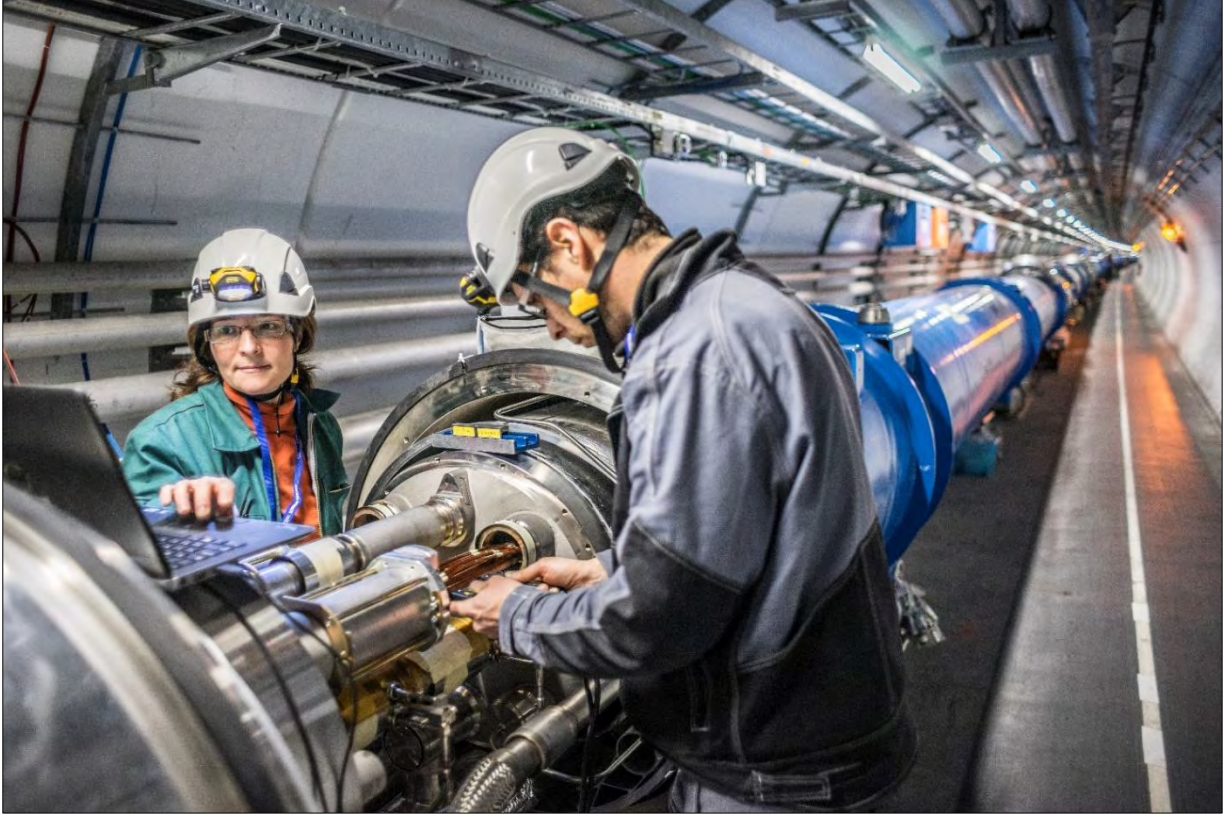
Figure 3: Technicians measuring on the connecting busbar between two magnets in the LHC tunnel (CERN, 2022g).
