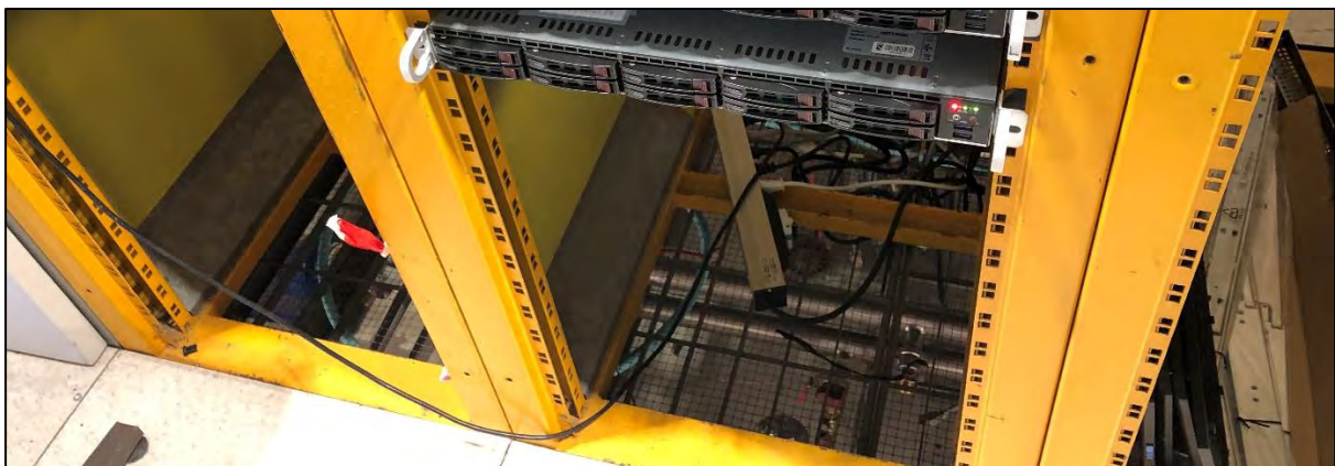
Figure 12: A rack where the grille can be seen at the bottom. Through the grille, it is possible to see the false floor and some of the installations also placed there (Own archive, 2022)
