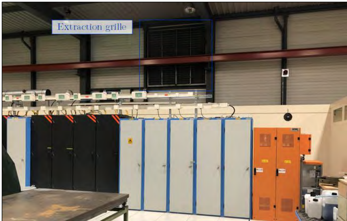
Figure 15: One of the recycled air extraction grilles places in the main hall (Own archive, 2022)
