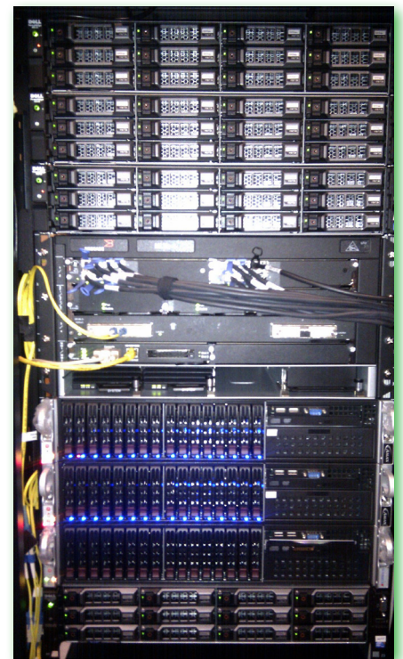
The equipment used by the Caltech team to break the data transfer record. Photo credit: D. Foster.
