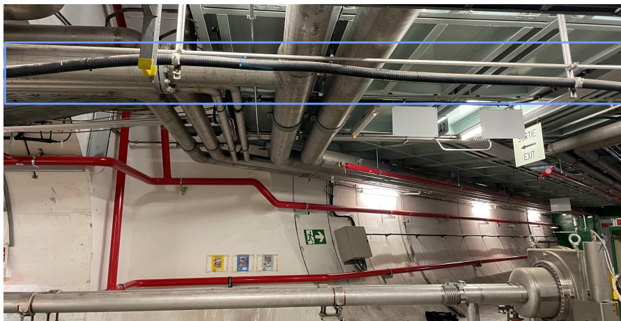
Figure 5.8: A plastic duct (highlighted inside the blue rectangle) was installed in the septum area to pull the oBLM. It is located at 2,36 m from the beamline approximately.
