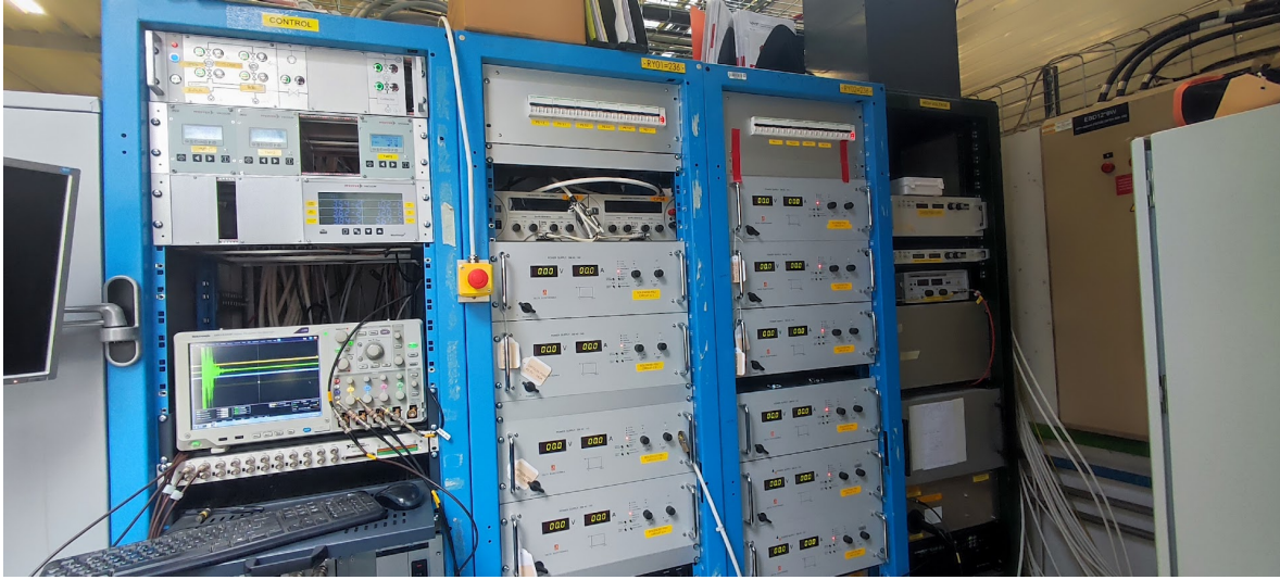
Figure 1.6: Four 19-inch control racks for EBTS with a locally connected monitor (left) for control and data access
