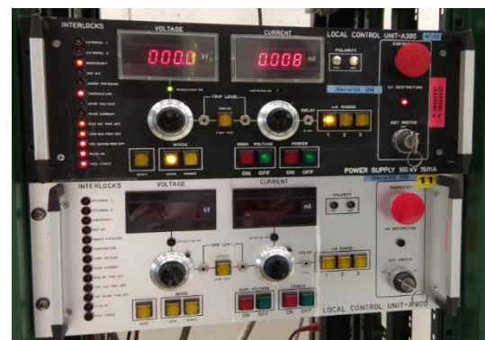
Fig. 37. 160 kV DC Power Supply
