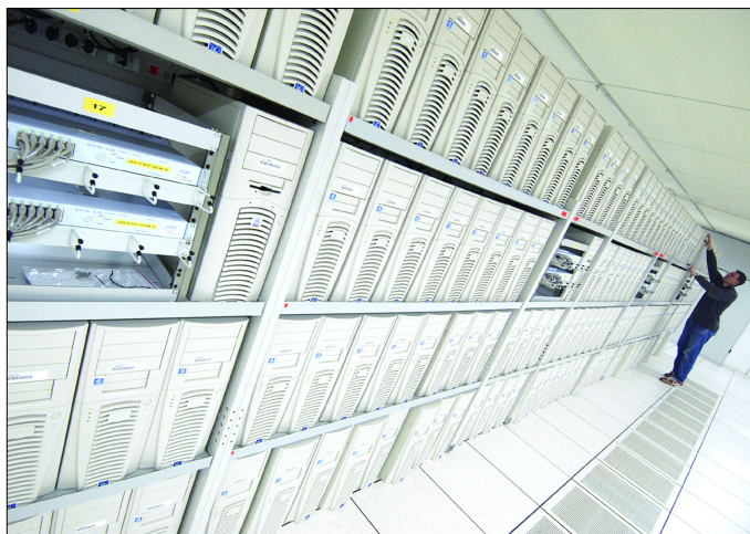
The new machine room in the basement of CERN's computer centre.
