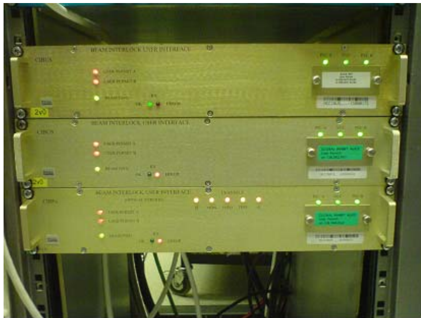
Fig. 4.8 CIBU modules for the user permits Beam (top), Injection 1 (middle) and Injection 2 (bottom). Two redundant lines (A, B), whose state is shown by LEDs, transmit the use permit flags to the CIBU. In this picture all permits are set to False.
