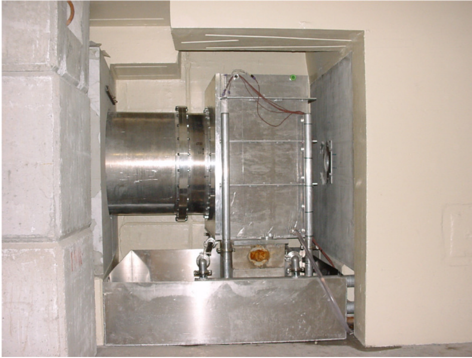
Figure 4.2: Pool containing the spallation target and showing the start of the neutron beam pipe
